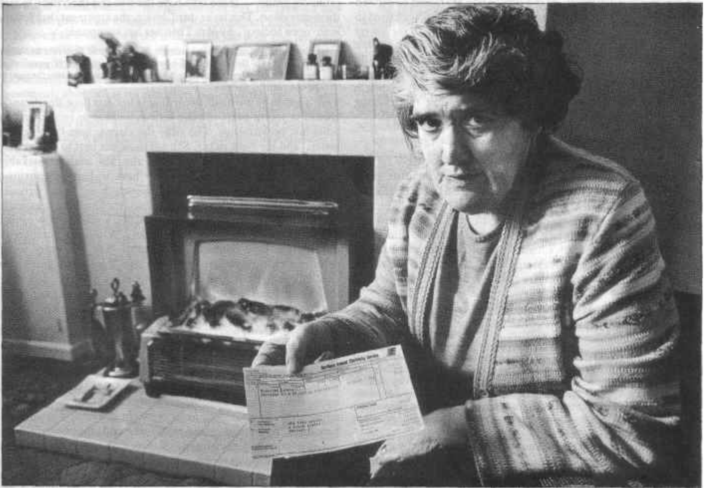
Mary Hughes from Belfast with one quarter's electricity bill for £272. When the house she lives in was redeveloped the Rayburn boiler was fitted wrongly, so she had to use her electric fire instead.
